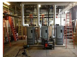
New Boilers Mean
